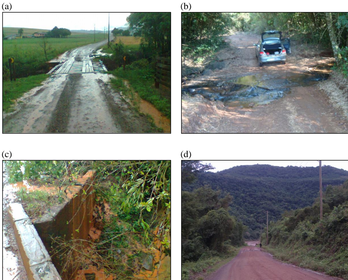
Figure 67 – Connections of unpaved roads with the tributaries (a, b) and the main river (c, d) in Guaporé catchment.
