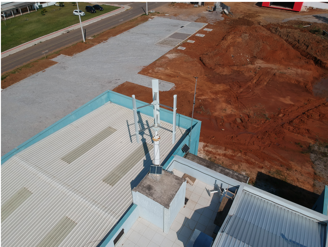
Figure 4.1 – Razec wind turbine.
