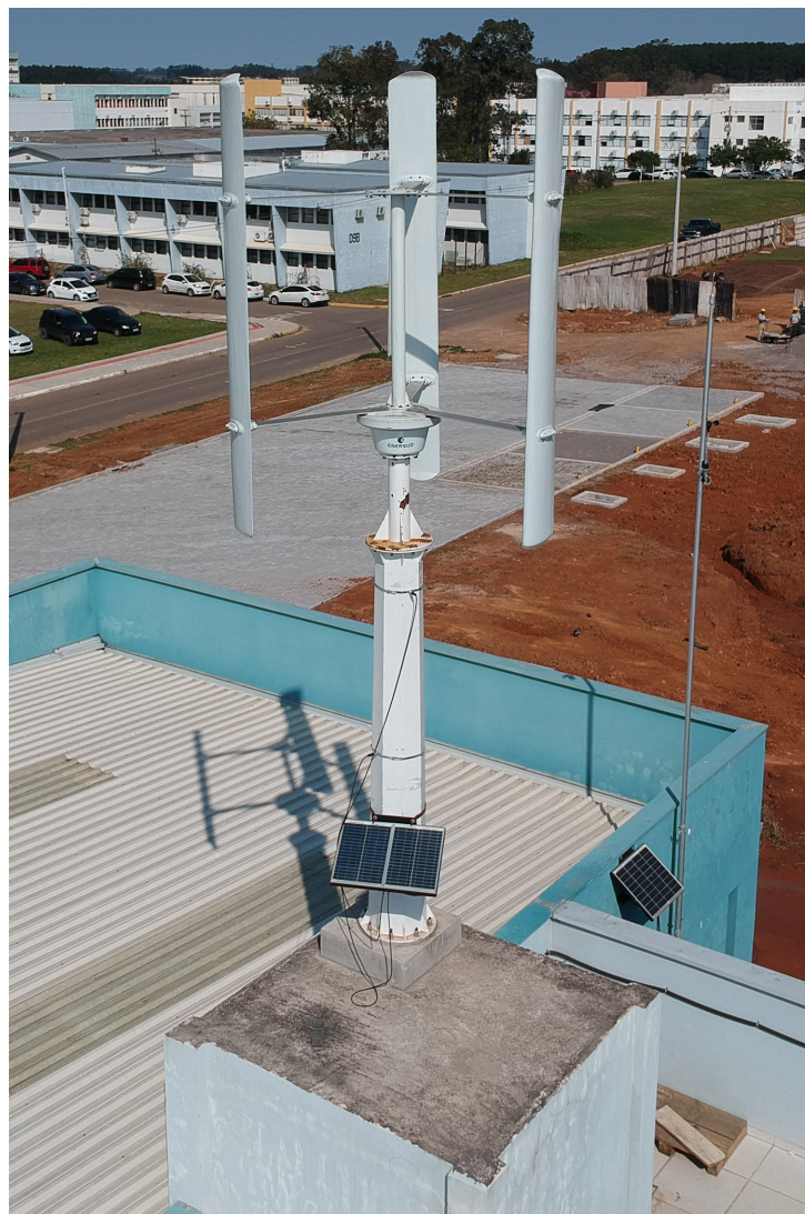
Figure 2.15 – Rooftop installed VAWT.
